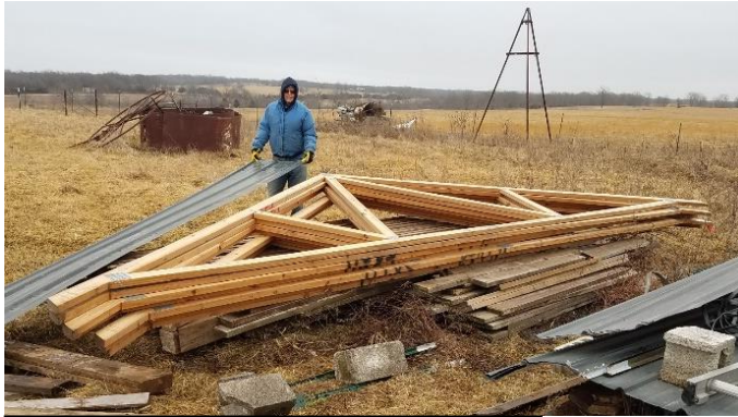
Trusses for the CCC Shelter House & Rick Hines with that Gleam in his Eye
